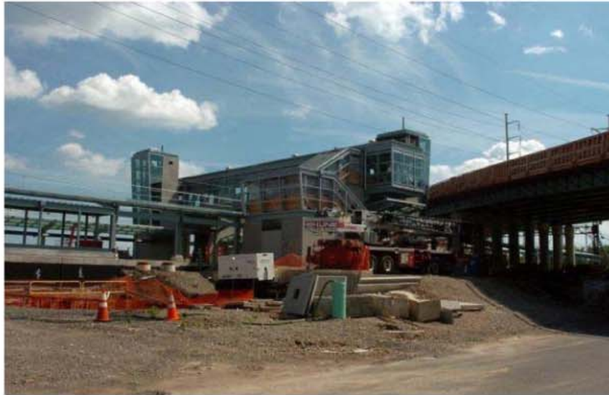
A view of the new Fairfield Metro Railroad station under construction, off of Kings Highway East in Fairfield, Conn. on Thursday July 22, 2010. Photo: Christian Abraham / Connecticut Post | Buy This Photo
